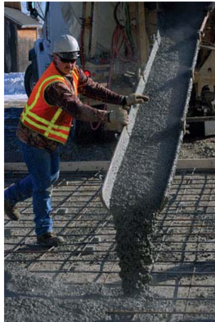
Jody McConnel of HC RediMix, Fairbanks, moves the chute to direct the flow of cold-weather concrete to create a concrete slab for communication and Stryker vehicle parking during a demonstration at Fort Wainwright March 26 and 27.
