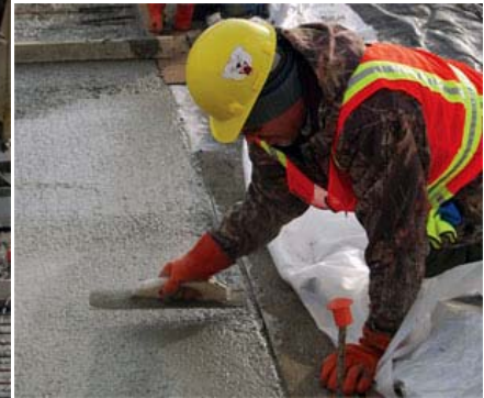
Finishers work a trowel over the solidifying concrete. This was the second year for such a project at Fort Wainwright, which incorporates cold-weather concrete, a technology developed by the U.S. Army Corps of Engineers' Cold Regions Research and Engineering Laboratory.
